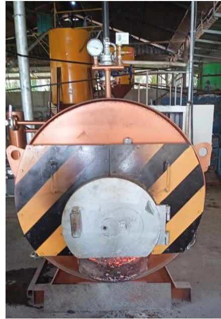
Boiler tampak belakang
