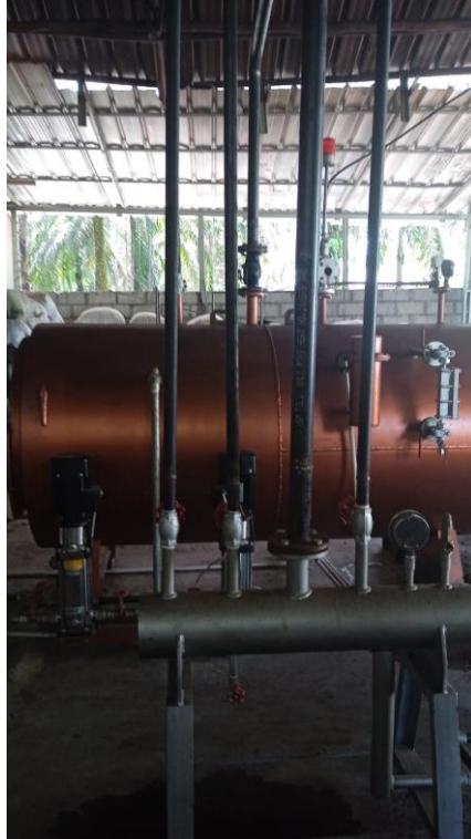
Boiler tampak samping kiri
