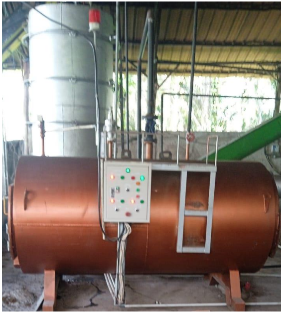
Boiler tampak samping kanan
